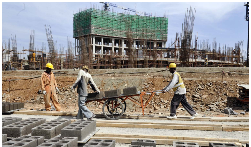
Construction works at the site of the new African Union (AU) conference center in Addis Ababa, Ethiopia. Photo : ANP/AFP
