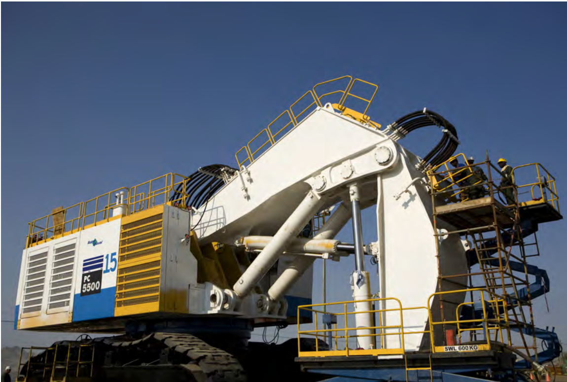
Mechanical shovel being assembled on site at the Rossing Uranium mine. Photo: World Bank, Flickr
